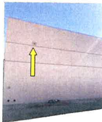
Photo 14 – Missing Light Fixtures West Side
